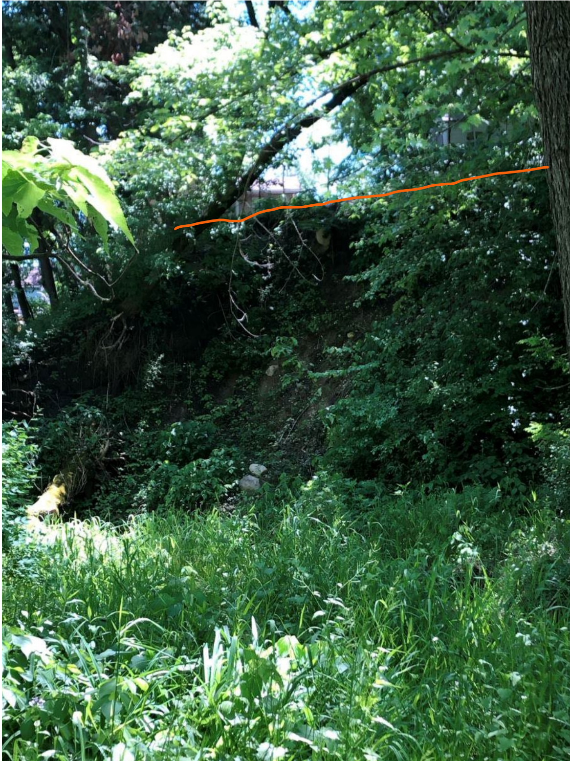
Figure 16. Spring Creek right bank and undercut bluff near 116 and 112 4th Street West (Site 3) from 416 Broadway; the approximate top of the bluff is highlighted in orange.
