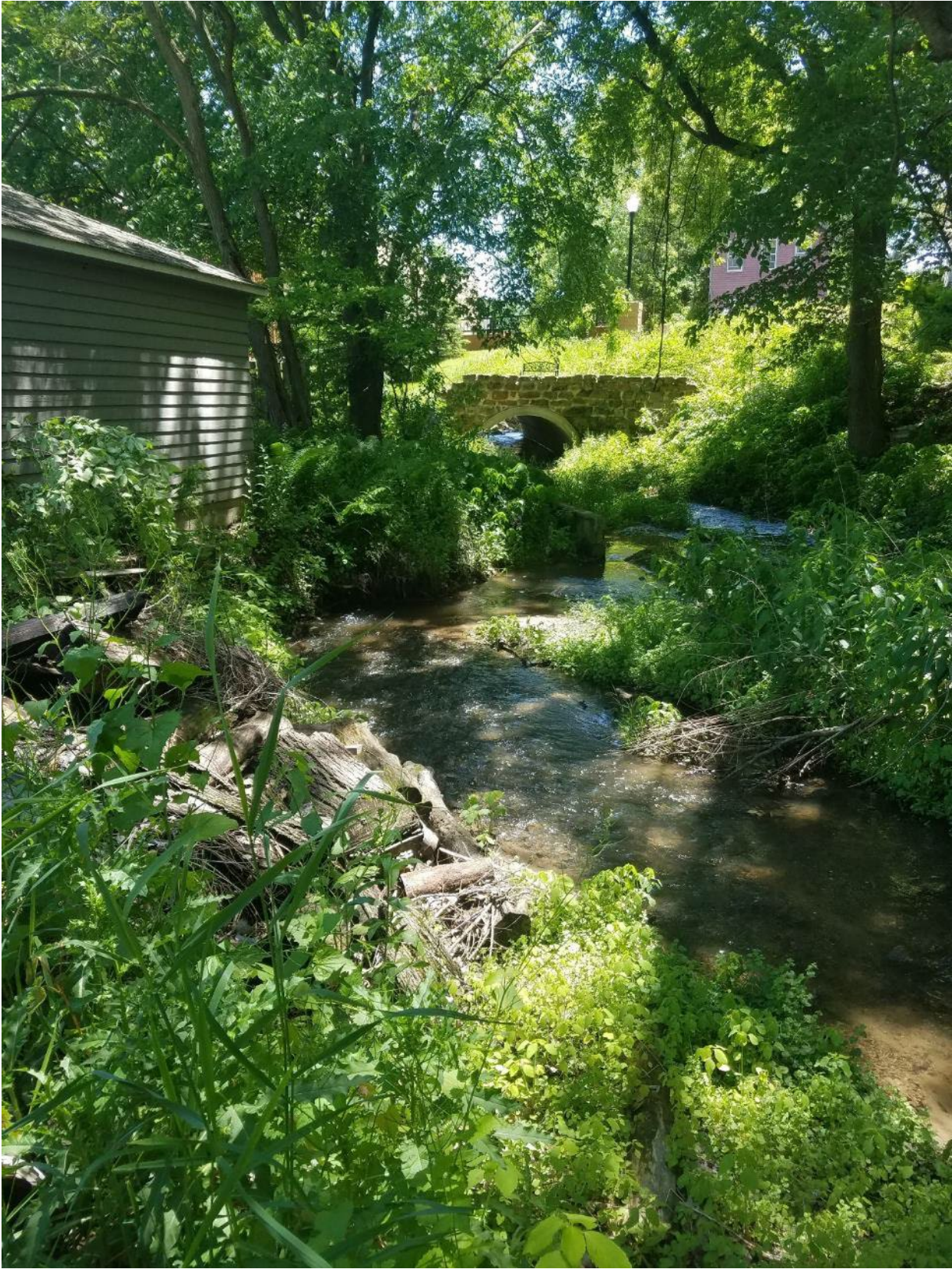
Figure 18. Spring Creek looking downstream at 404 Broadway accessory structure and debris pile on the left bank.
