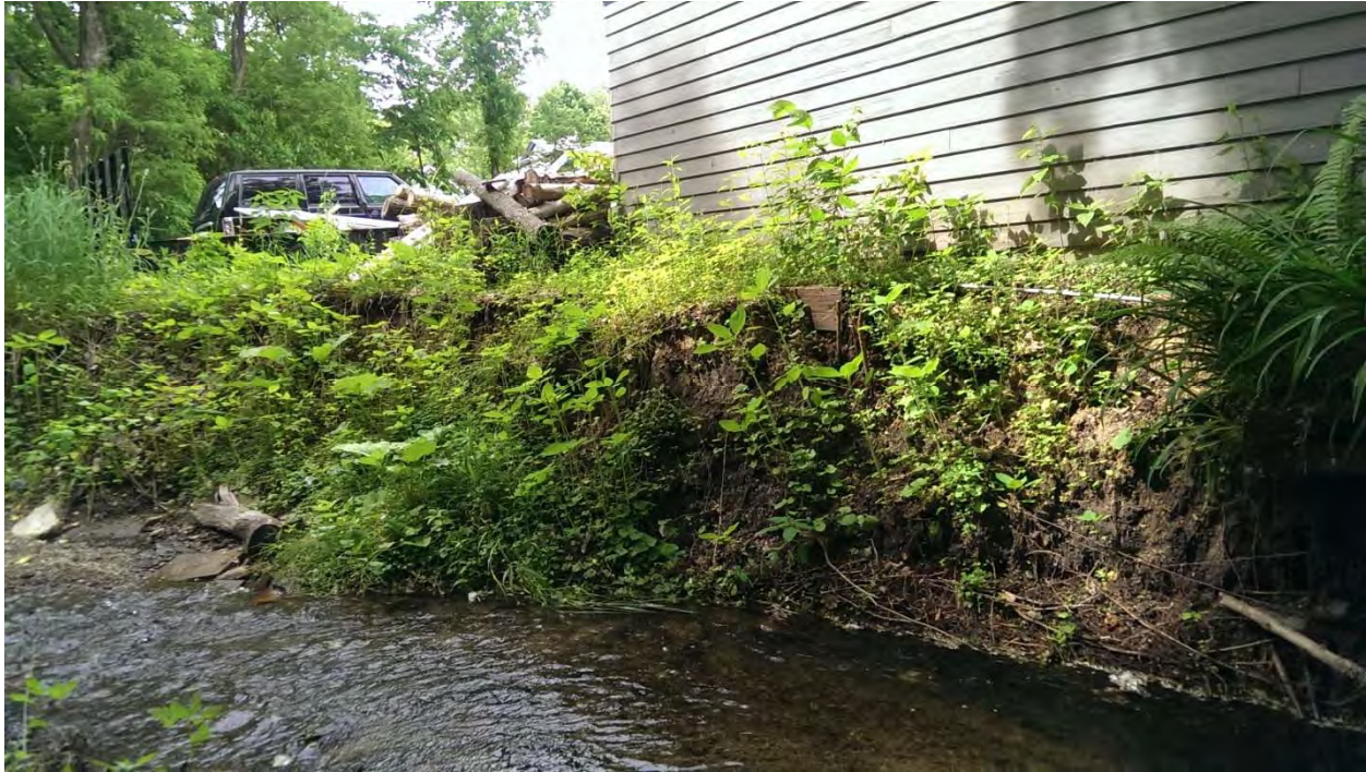
Photo 9: Close-up of recent erosion that is within a foot or two of the homeowner's garage
