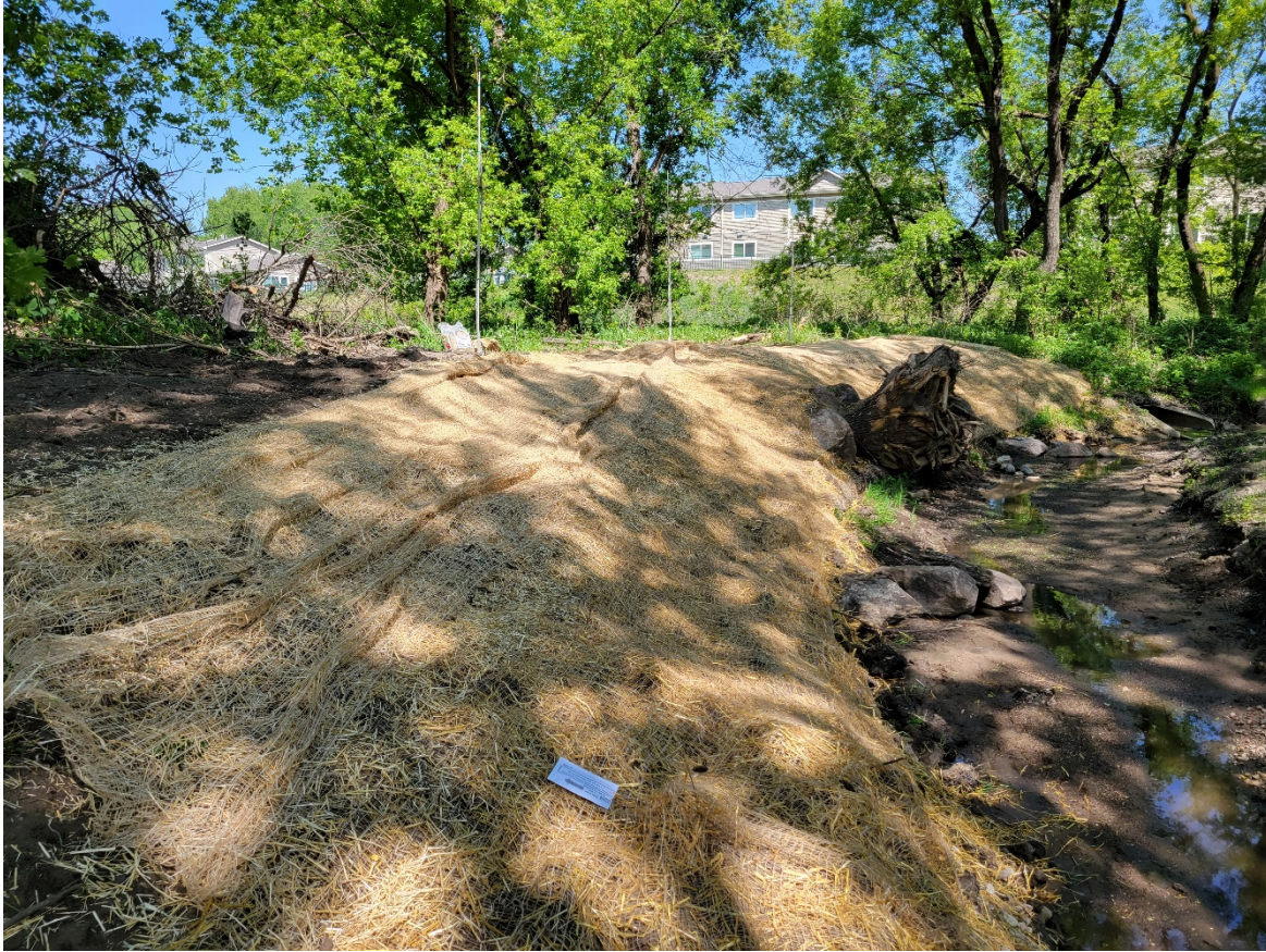
Cut back steep slope near large root wad station 8+30, seeded and added blanket
