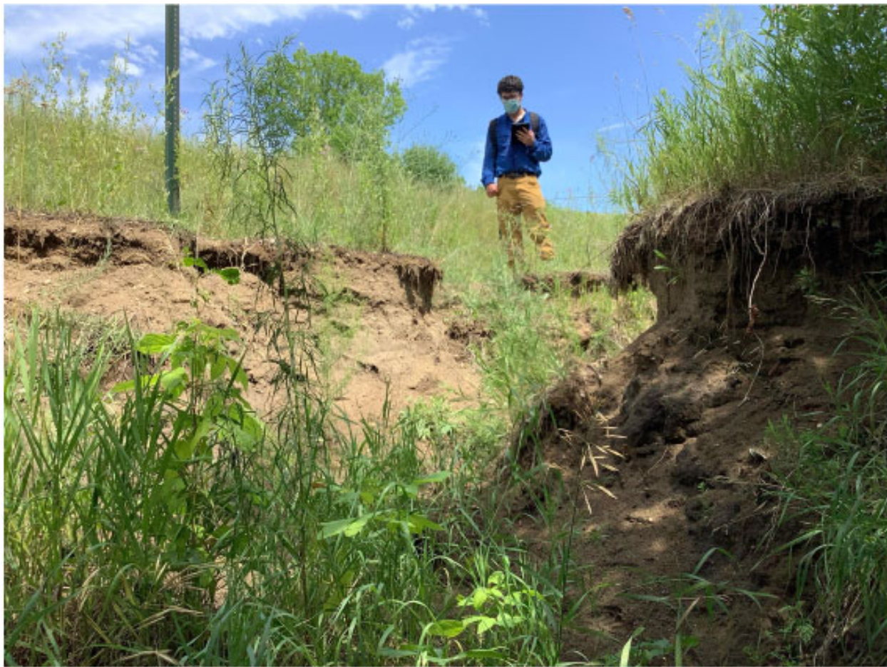
Figure 104. View of Gully 999-105 taken in 2020 looking upstream toward the pedestrian walking trail and gully head cut.
