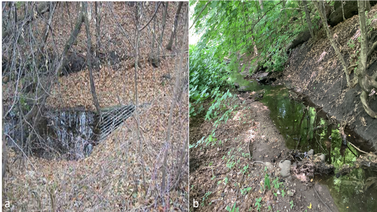
Figure 66. Photo 'a' is an image taken in 2008 of the culvert forming the head cut of L178 and its downstream channel; Photo 'b' is an image taken in 2020 of L178's downstream channel, showing significant incision of the channel.
